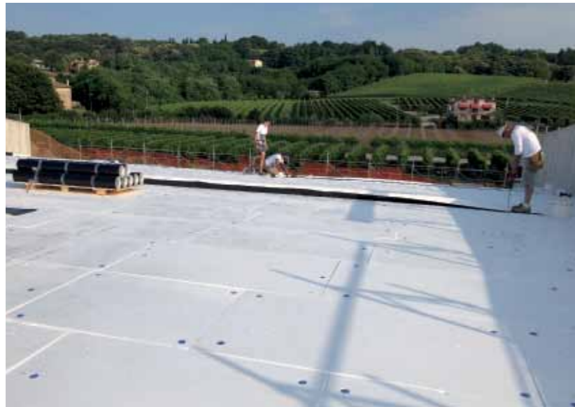
ABOVE. Application of Mapeplan T B synthetic membrane over the insulating layers.
